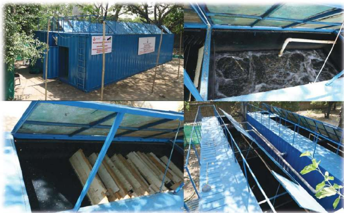
Figure 74 Package sewage treatment plant installed in a residential complex in New Delhi
